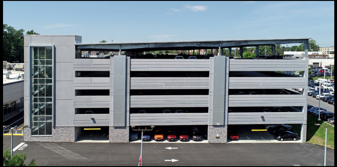
Parking Garage Solar Canopy is 55,076 sf on the fifth floor and generates 891 KW solar power. It provides 83% of the electrical requirements for Fitzgerald's Auto Mall in Gaithersburg.
