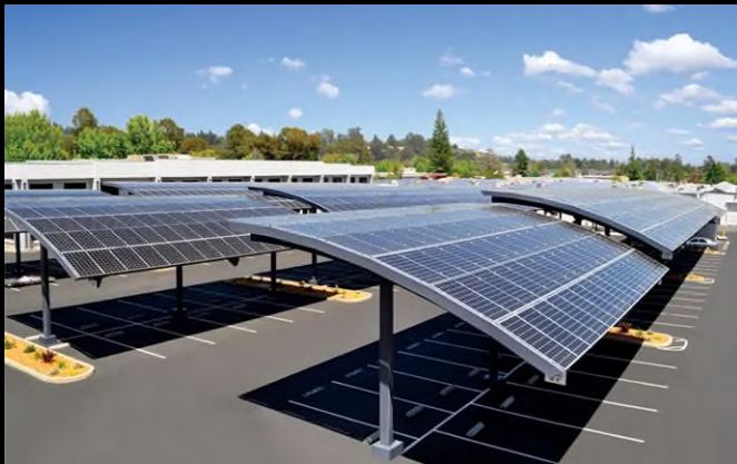
Solar Canopies for Parking Lots
