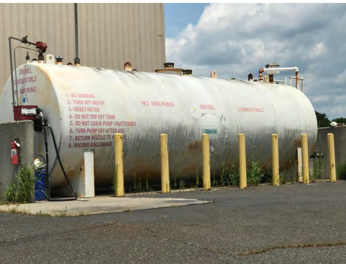
10,000 Gallon Diesel Tank
