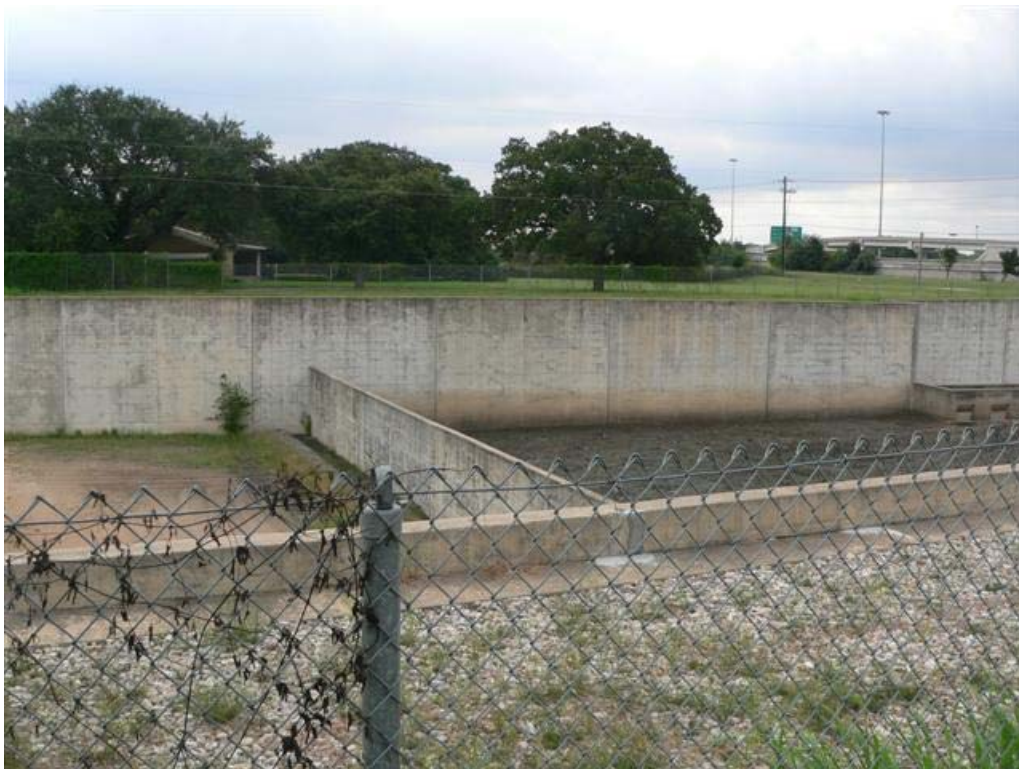
Photo No. 12: View of water quality basin located to the west of the Subject Property next to the residence.
