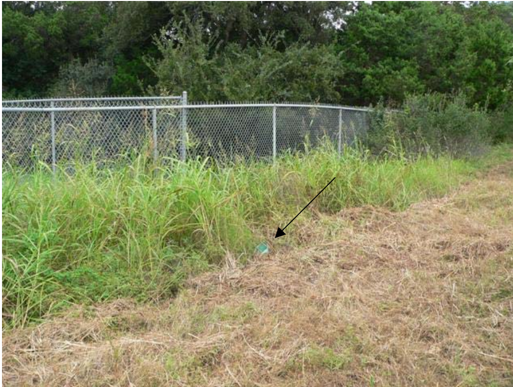
Photo No. 5: A 6-inch PVC pipe was observed along the western property boundary and appeared to be associated with the sanitary sewer line.
