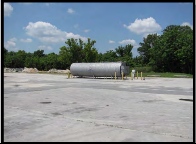
Diesel Fuel Tank
