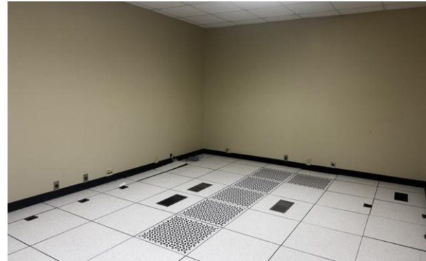
Special-Use Room with Raised Floor
