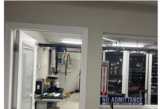
1000sf data center infrastructure
