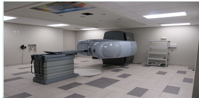
Shielded procedure / treatment room
