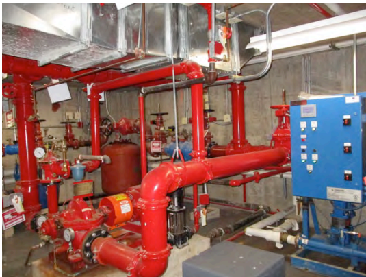
1 ST FLOOR WATER PUMP SYSTEM
