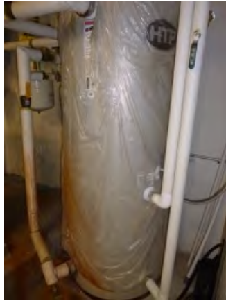
1 ST FLOOR HW HEATER
