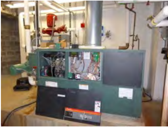
1 ST FLOOR CHURCH MECHANICAL ROOM
